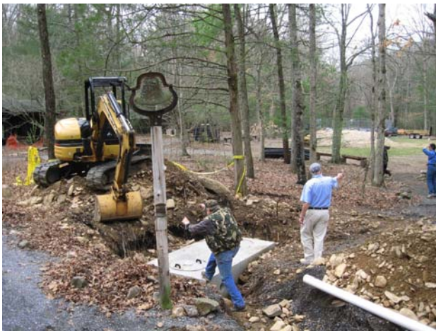
Heavy machinery on site to begin the trenching for new pipes and electrical wires.
